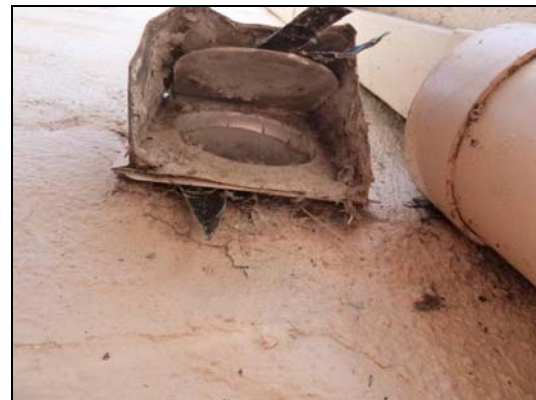
Vent damper does not close
