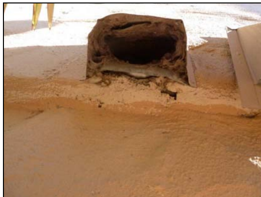
Vent needs cleaning so damper can close
