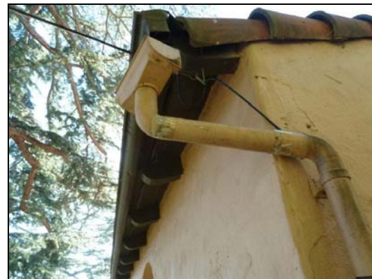
Down spout does not line up with gutter
